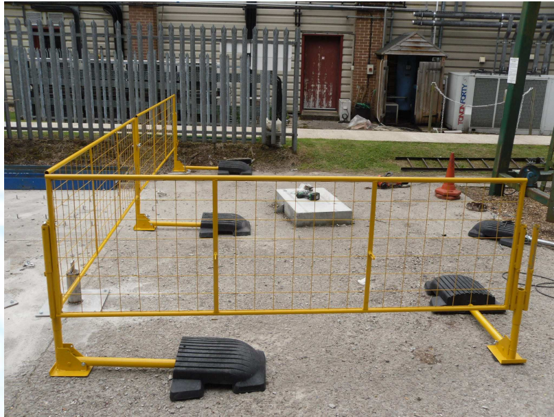
Figure 2 – Temporary edge protection system including corner
